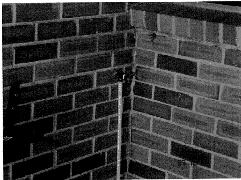
Photo 12: Exterior Hose Bibb
